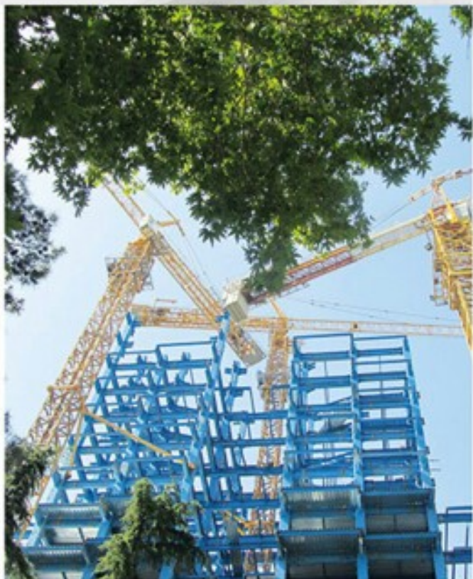
Fabrication and Erection of Steel Structures of Residential Buildings in Tehran, Zafaranih / 570 TON
