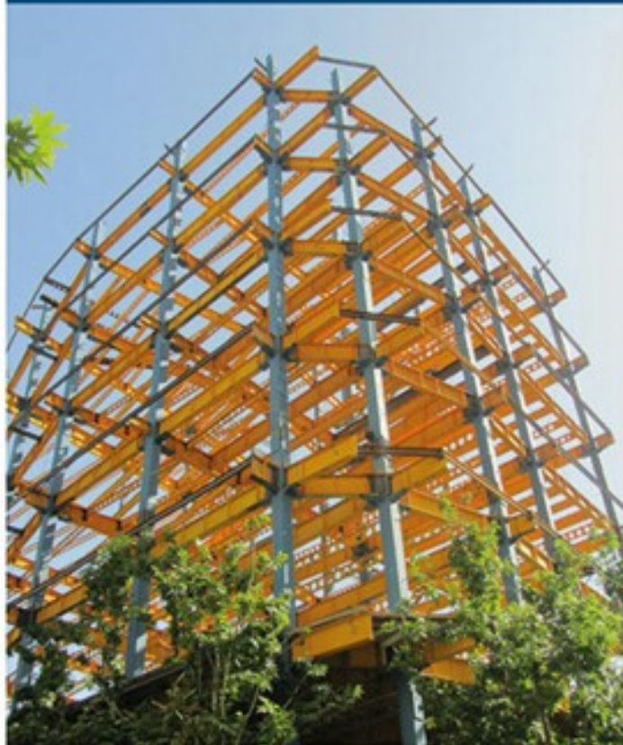
Fabrication and Erection of Steel Structures of Residential Buildings in Tehran, Niavaran / 370 TON
