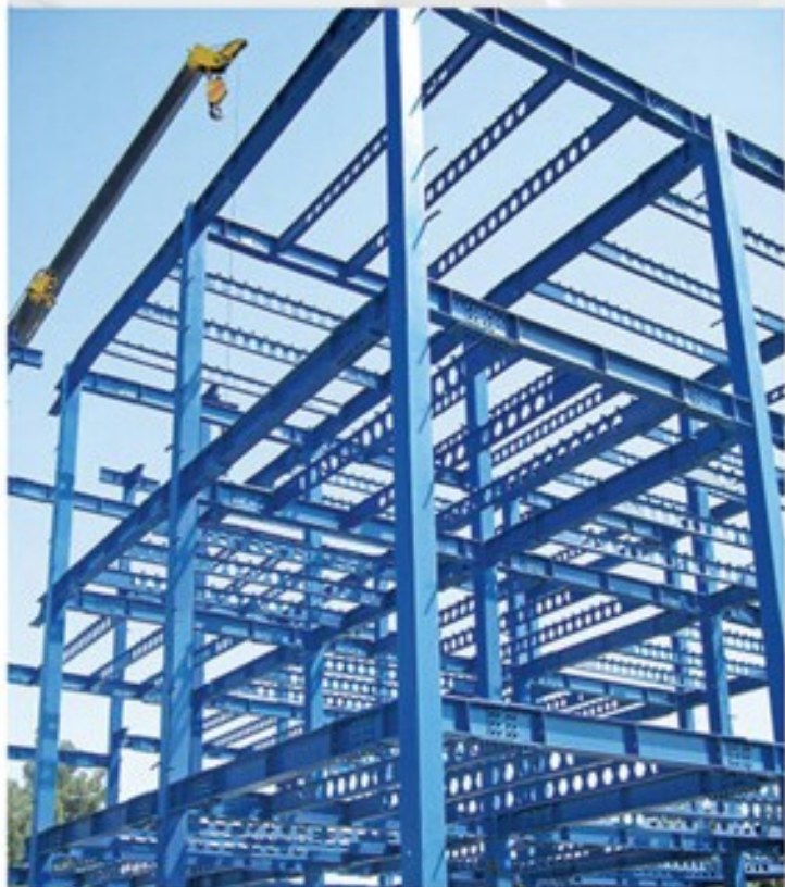
Fabrication and Erection of the Steel Structures of the Office Building of Alifard Company (Sun Ich) / 360 TON
