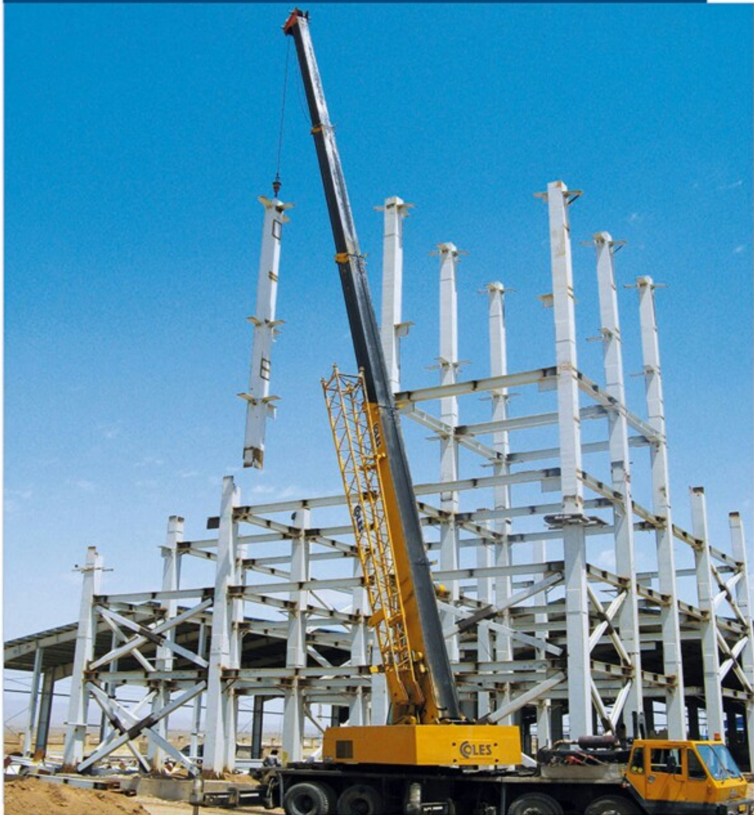
Fabrication and Erection of the Steel Structures of Thermal Ceramic Company / 1200 TON
