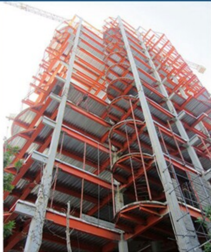
Fabrication and Erection of Steel Structures of Residential Buildings in Karaj / 550 TON
